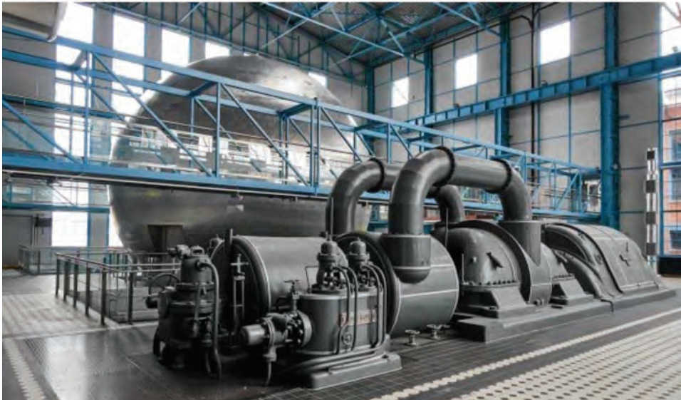
Photo 1. The historic power generator in the power station EC1, Lodz, 14/33 Kilinskiego Street, September 2015, photo by W. Kazimierska-Jerzyk
